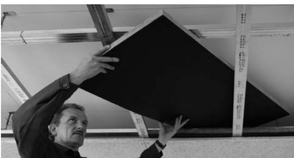
Insertion of Heralan absorber panels one by one along with the installation of the Heradesign panels. Panels that get jammed between the sections are cut to size.
