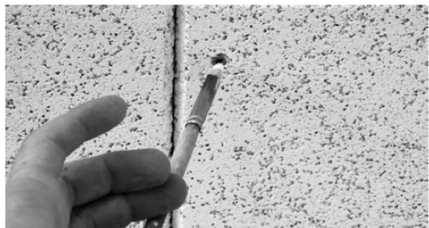
Paint over the screw heads with the supplied paint or an equivalent one. The screw heads must be flush with the surface of the panel.
