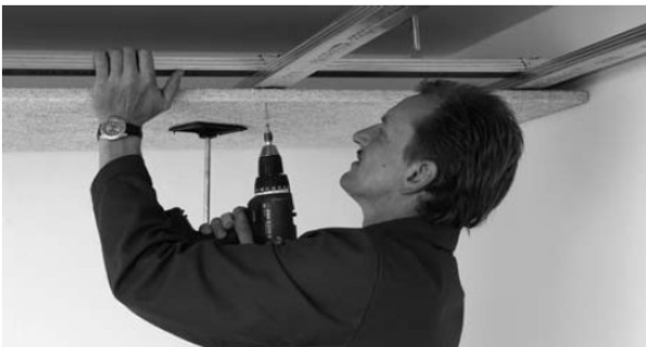
Installing the panels by means of supports. Press the panel onto the section with the ball of the hand while screwing. There mustn't be a gap between the panel and the section. Only work with the panels with clean hands and a clean tool.
