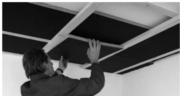
Insertion of Heralan absorber panels one by one along with the installation of the Heradesign decorative panels. Panels that get jammed between the wood laths are cut to size.
